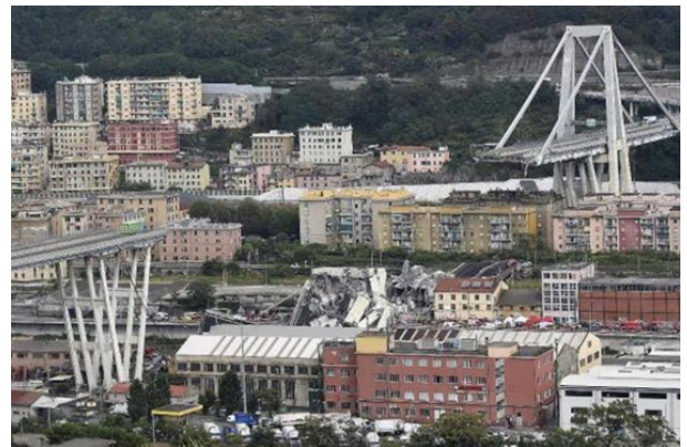
Figure 4- View of the Morandi Bridge after the collapse occurred in August 14, 2018 due to the downfall of a cable stay which dragged down the repaired piles number 9
