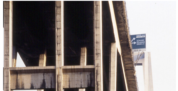
Figure 1- Damaged reinforced piles withstanding the roadway of the Morandi Bridge in 1979
