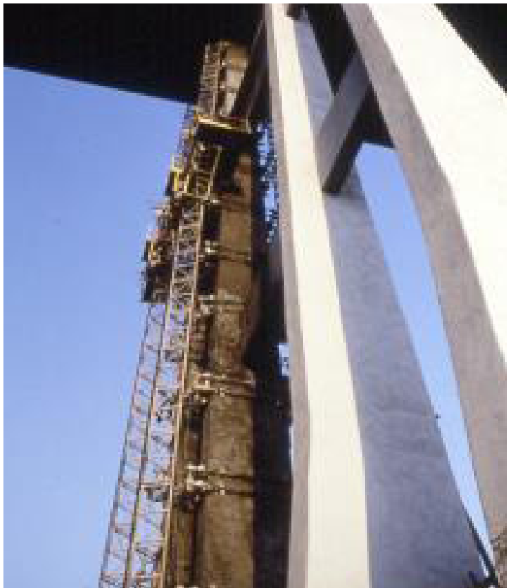
Figure 2- On the left hand a pile is shown during the spraying and floating of the repairing mortar; on the right hand two piles are shown completely coated by the white flexible paint
